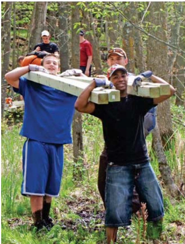
Two young volunteers help carry the load at Straight Lake State Park in Polk County. Volunteer trail builders carried all the lumber, hardware and tools to build a 400-foot boardwalk, and they carried it over half a mile. Some volunteers did nothing but carry lumber. Photo by IATA Board member John Helling of Luck, WI.
